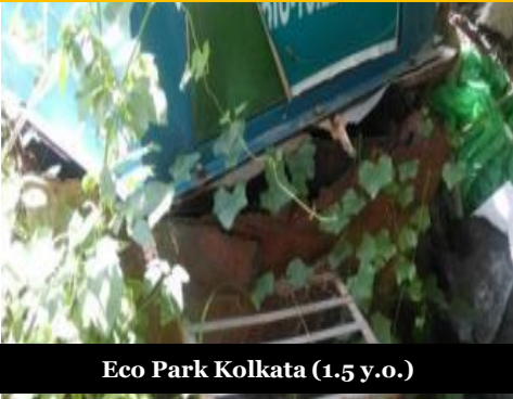
Structure Foundation Rusting
