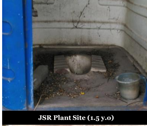
Broken Non-usable Unit
