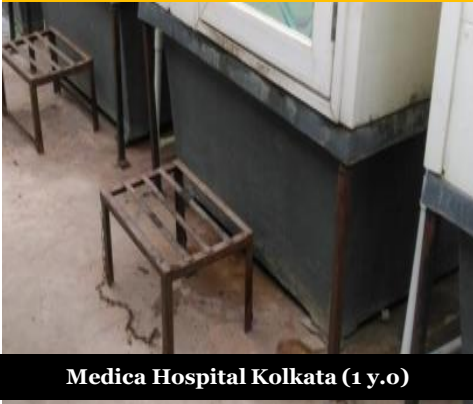
Structure stand rusting
