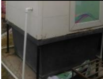
Water Pipes prone to damage
